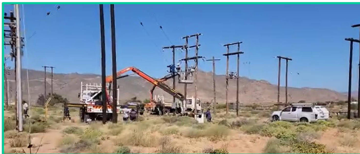
Picture 17: Electricity transformer installation
