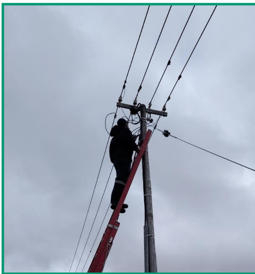
Picture 7: Supporting electrical infrastructure
