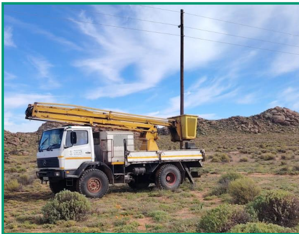
Picture 19: Supporting electrical infrastructure
