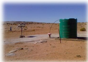
Sun panel with green tank
